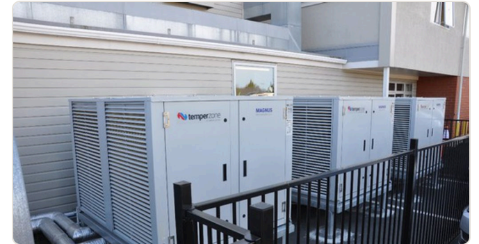
The space heating machines as installed. Photo from the published report.
